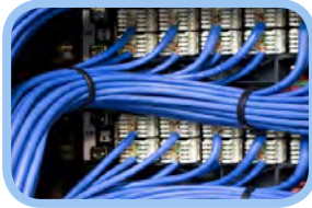
DCT Fibre Optics & Data Centre Solutions
