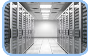
DCT Data Centre Design
